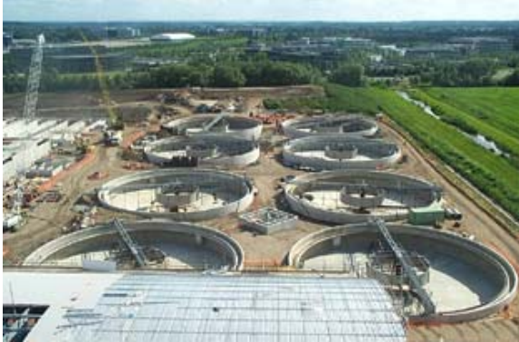
The Reading sewage treatment works was one of the first projects to be assessed under the CEEQUAL scheme. The project achieved an 'Excellent' Award.
