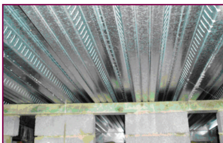
Galvanised steel decking forming the underside of a ground floor slab after 10 years
