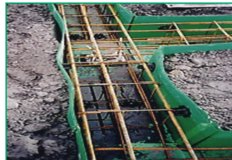
Figure 1 Lack of specified cover to reinforcement.
