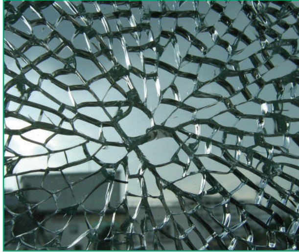
Nickel sulfide failure of toughened glass (courtesy of Sandberg)
